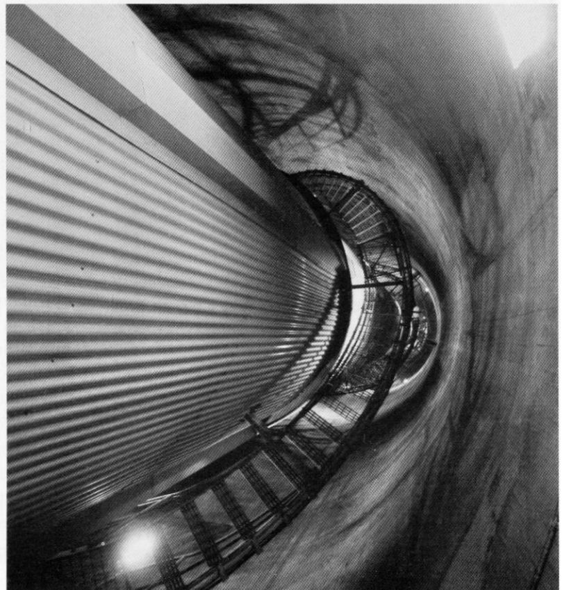
The bottom end of the huge exhaust pipes. Daylight can be seen far up. These four exhaust pipes are the only part of the power station that are above ground.
